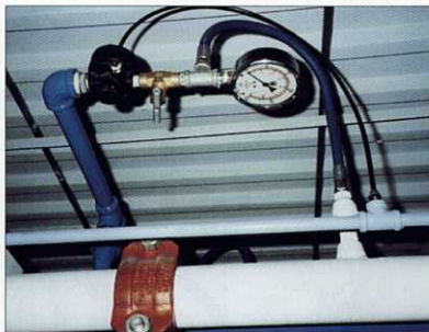
Air injector installed on conveying line
