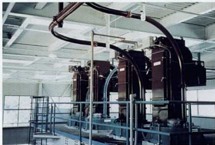
Compound ingredients are fed through a rotary valve and carried by the dense-phase pneumatic conveyor to the appropriate receiving bin. Pictured are the tops of each receiving bin.
