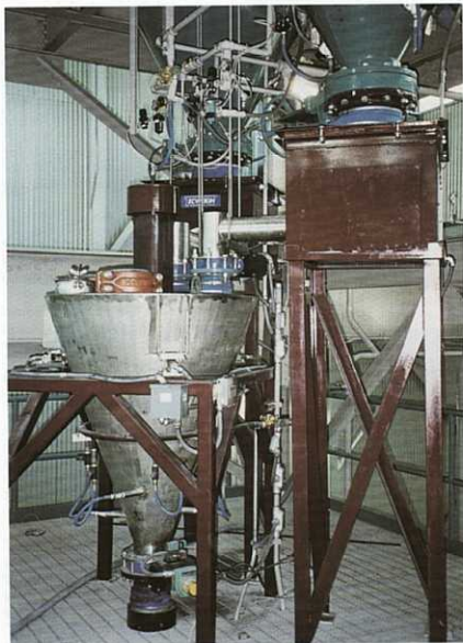
A screw feeder delivers compound ingredients from a receiving bin into a weigh hopper, which discharges into the mixer.
